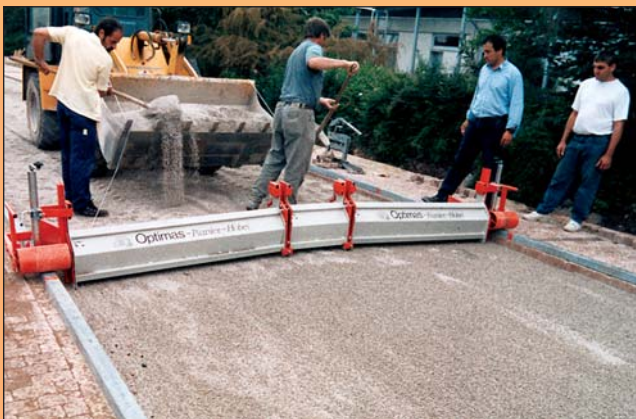
Final layer of sub-base ( fine stone chipping) and crown for water drainage are prepared in one stage.
