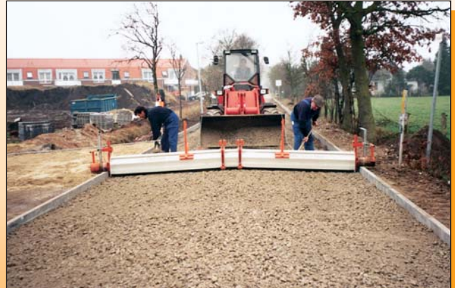
Sub-base layer of coarse gravel mixture and crown for water drainage are prepared in one stage.
